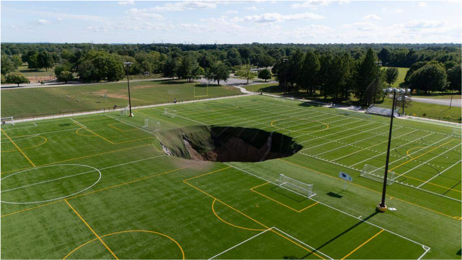
A sinkhole in Gordon F. Moore Park in Alton, Ill. on June 26, 2024 after an old mine collapsed and brought down a field light. Joshua Carter Belleville News-Democrat
